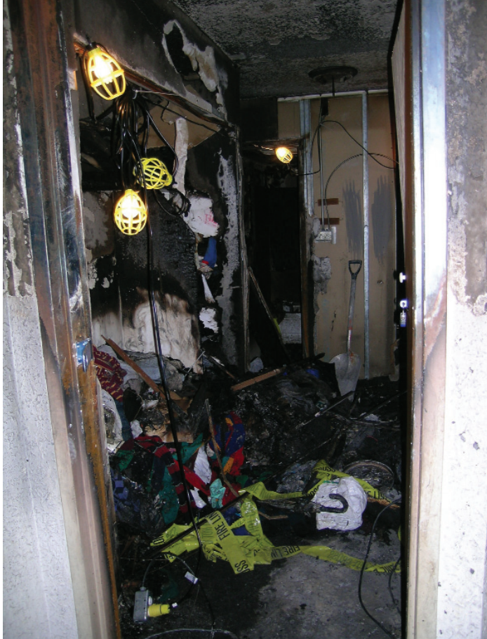
Figure 6. Debris resulting from a building fire. This material is a highly heterogeneous collection of contents, furnishings and furniture, and building material. Debris from building fires can contain soot, partly-burned particulate material to which PAHs are attached and possibly chlorinated dibenzofurans and dibenzodioxins. This debris also can contain asbestos-containing materials. The presence of asbestos-containing materials depends on the age of the building.
