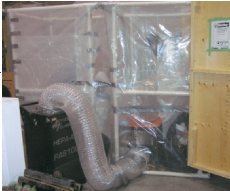
Figure 1 (Opposite page): A HEPA-filtered vacuum cleaner serves as both negative airmover and vacuum cleaner. Note the location of the vacuum cleaning machine and its discharge outside the containment.
