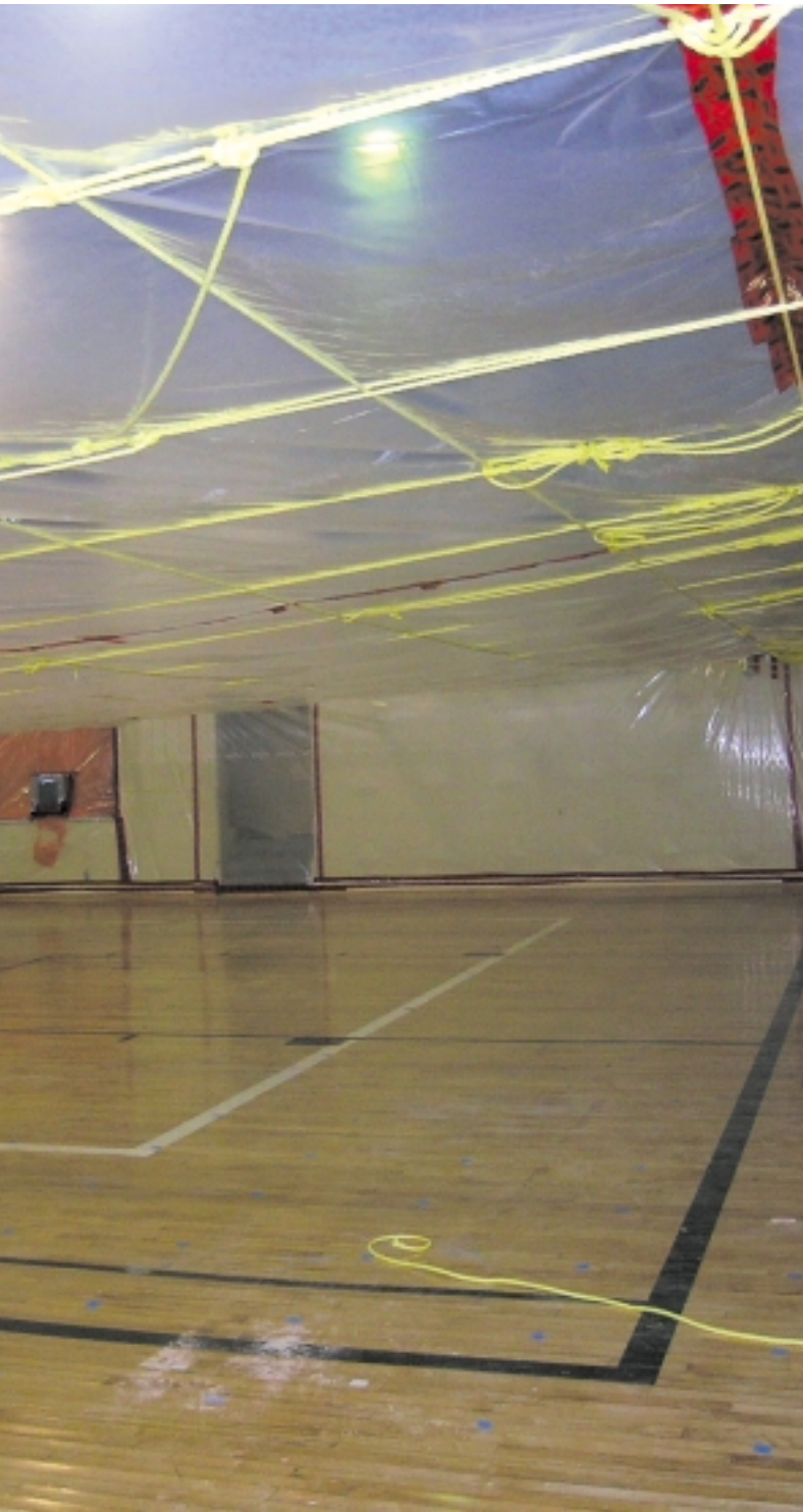
Macro containment showing the sag in the ceiling due to negative static pressure.
