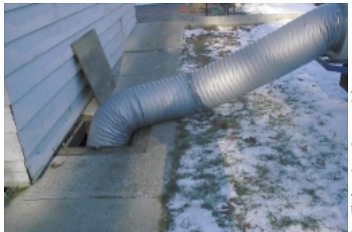
Figure 3. Heated air provided to the crawlspace.
