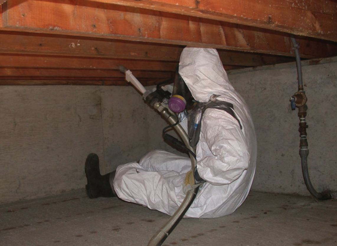
This picture depicts the work posture in the crawlspace. The speed of the work, compared to sanding, compensates somewhat for the lack of ideal work position. Note the position of the probe of the four-gas tester on the shoulder of the worker.
